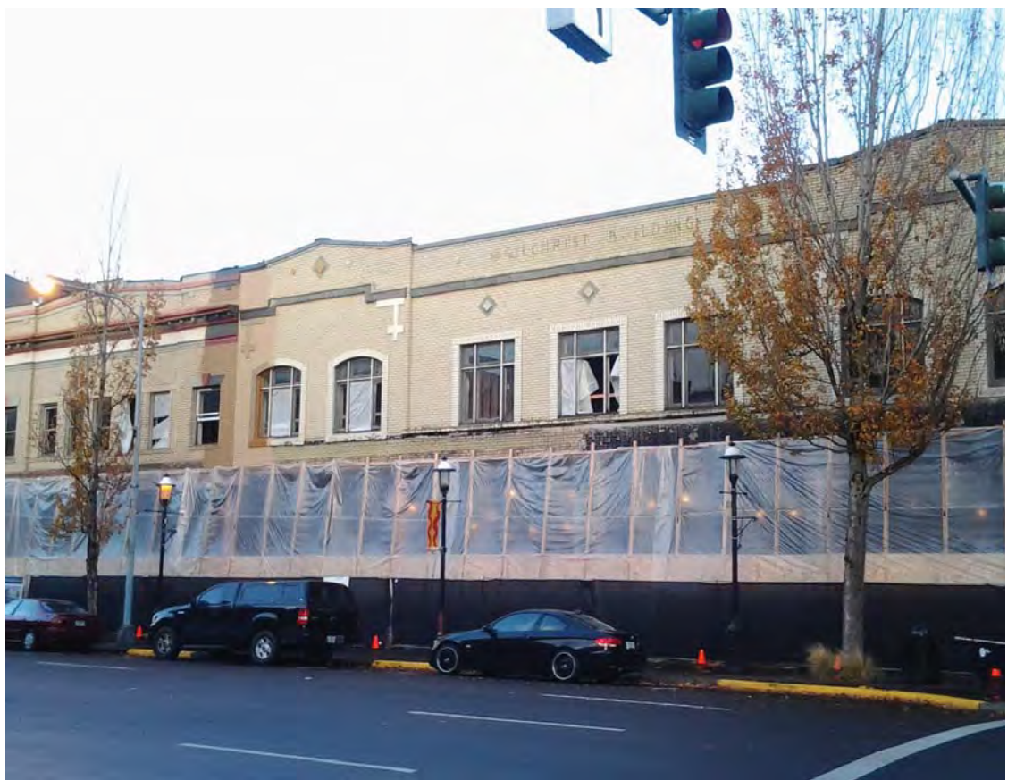
The McGilchrist building is being restored to make room for several businesses and apartments. The project is expected to open in early summer.
