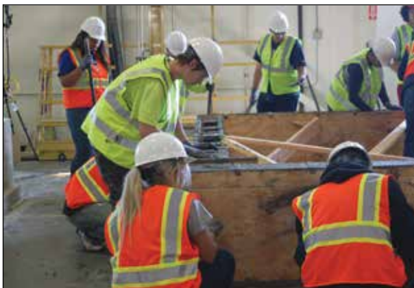
Below: CTEC students working with cement to build the foundation of a project.
